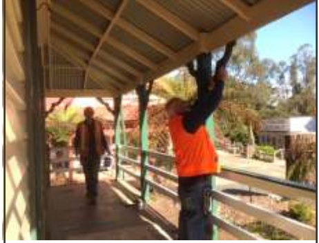
(above & right) Friends of Coal Creek volunteers hard at work repairing the Auctioneers Rooms
